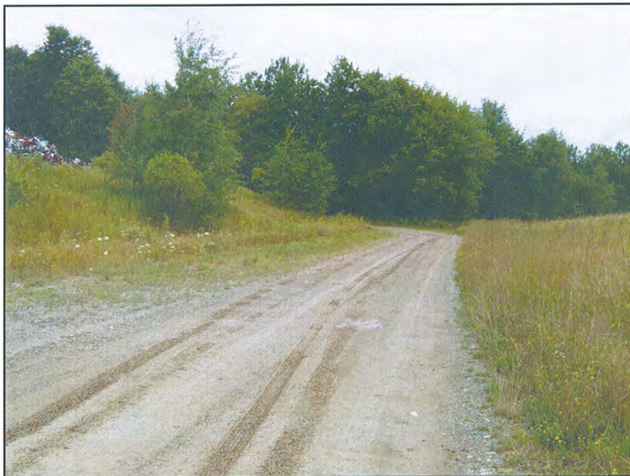
Photo 14. Disturbed - Access Road
